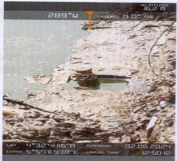
Incident point with 2" valve installed.
